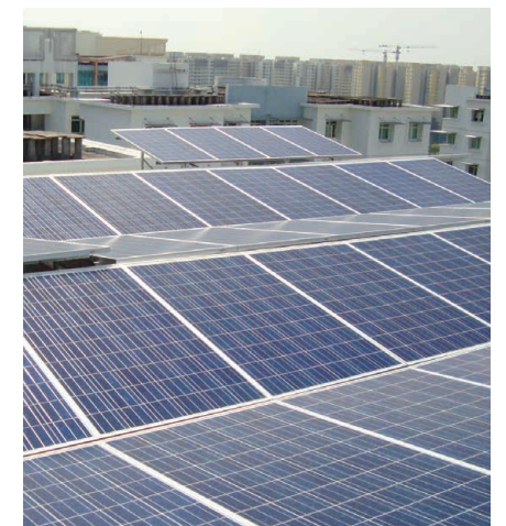
Solar panels installed atop HDB blocks
