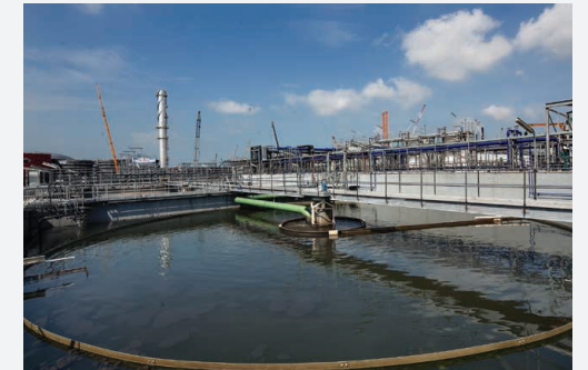
One of Sembcorp's wastewater treatment facilities on Jurong Island
