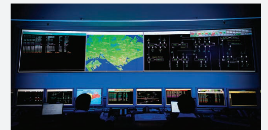
SP's SCADA (Supervisory Control and Data Acquisition) system monitors and controls the national grid, and is one of the systems that the SP Centre of Excellence will look to enhance with next-generation technologies.
